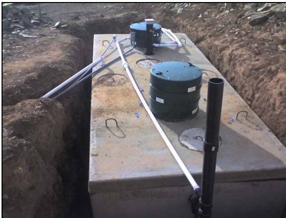
Single concrete tank with risers & supply/return lines to dripfield (the Hoot BNR tank measures 13'6" L x 6' W x 6' H)
