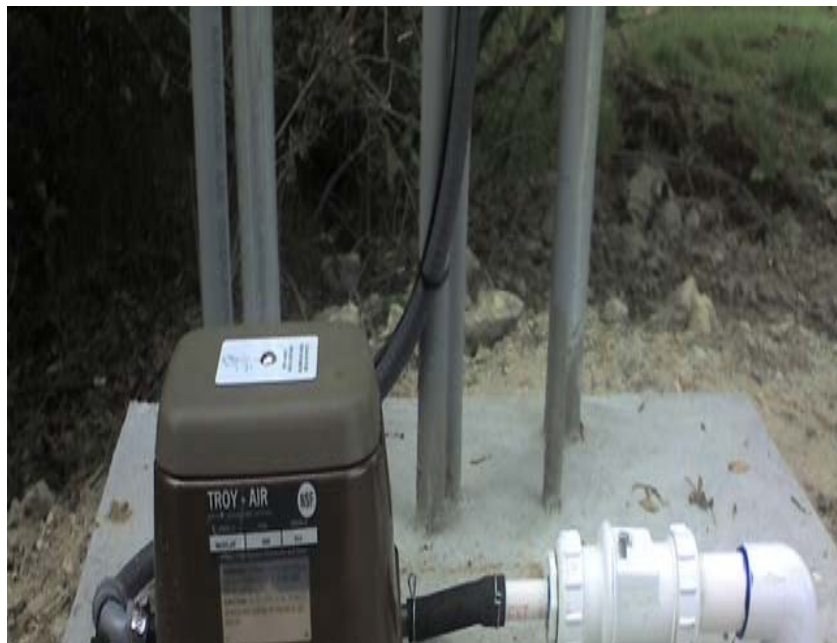
Blower with check valve and rubber hose connections — 1- \frac{1}{4} " PVC line back to tank aeration manifold
