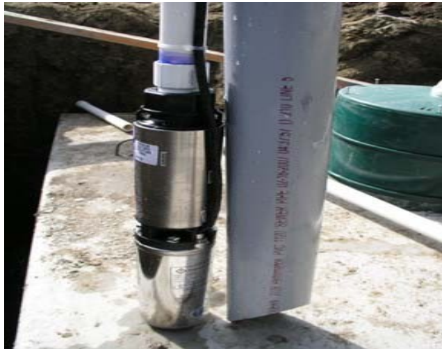
Pump prep — 1- \frac{1}{4} " male adapter installed with Teflon tape, PVC pipe attached, power cord tied with Ty-rap
