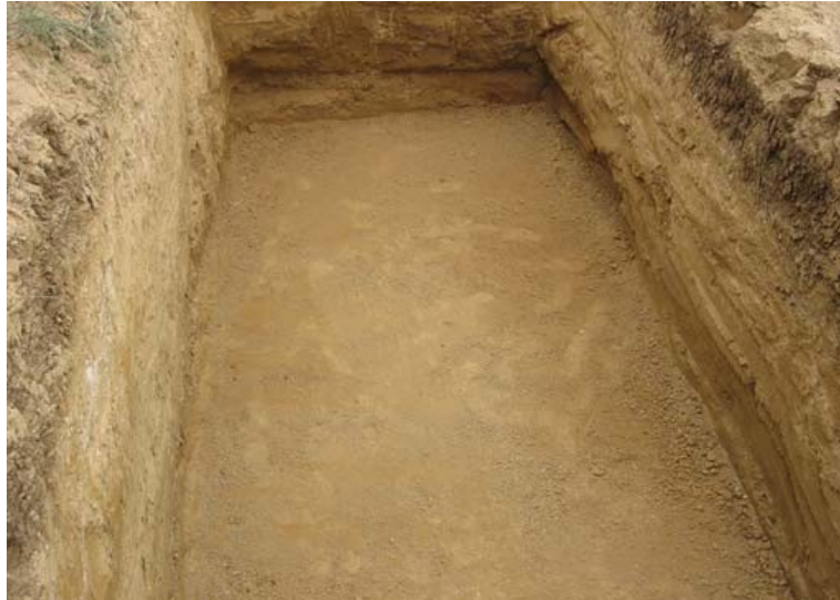
Properly excavated and graded tank hole — smooth, level, free of sharp rocks
