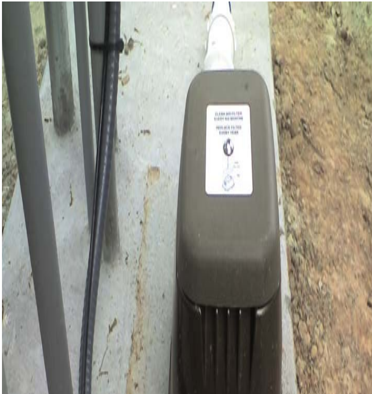
Blower with liquid flex conduit installed for cord protection
