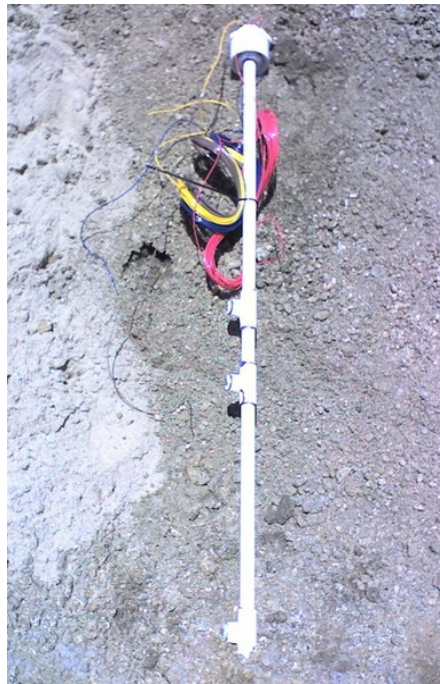
Hoot sensor probe assembly — installed and connected by SOS
